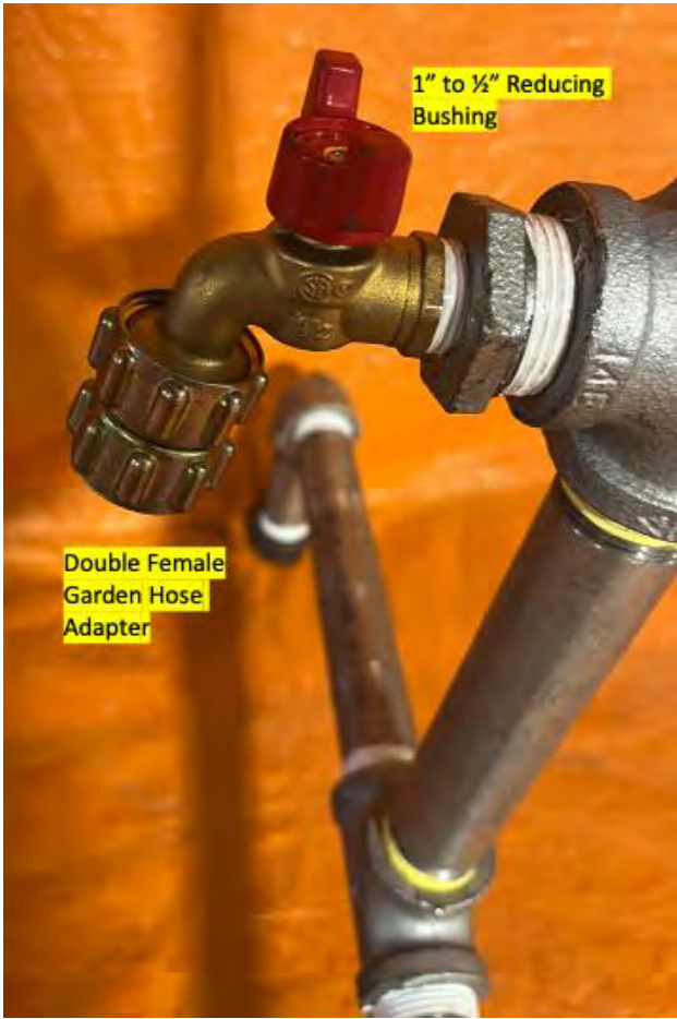
Pipe Stand Patch and Valves
