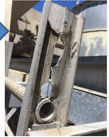
Sheared Metal Ladder
