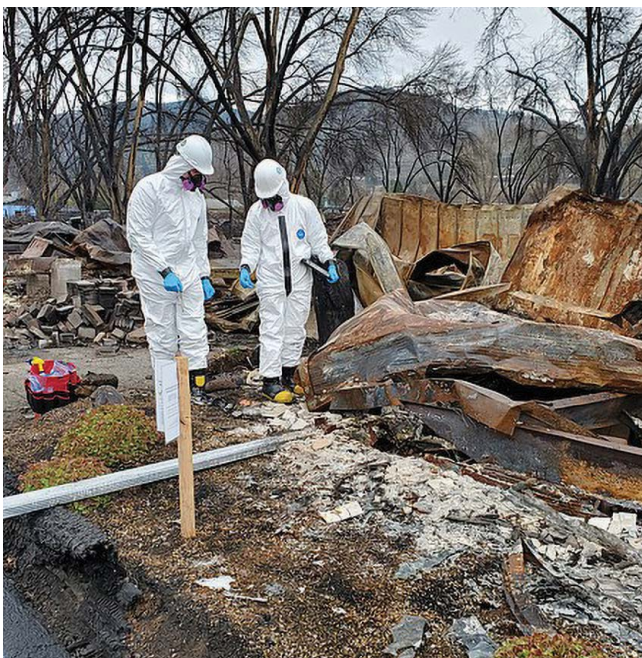
Wildfire cleanup in Almeda, Oregon. (Photo courtesy of Oregon Department of Transportation).
