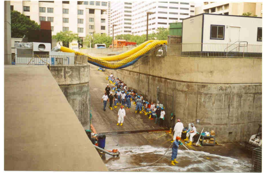
Flooded loading dock after pumping
