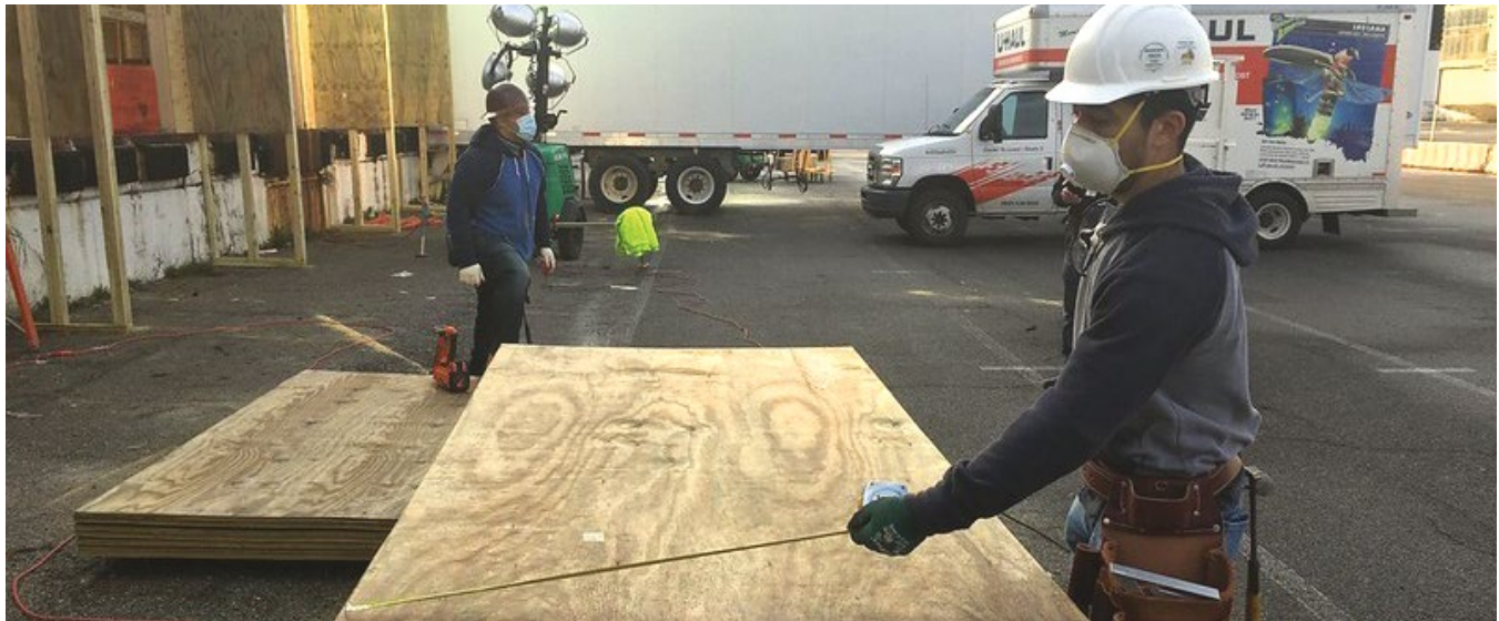
Carpenters working during the COVID-19 pandemic. (Photo courtesy of New Jersey/New York Hazardous Materials Worker Training Center).
